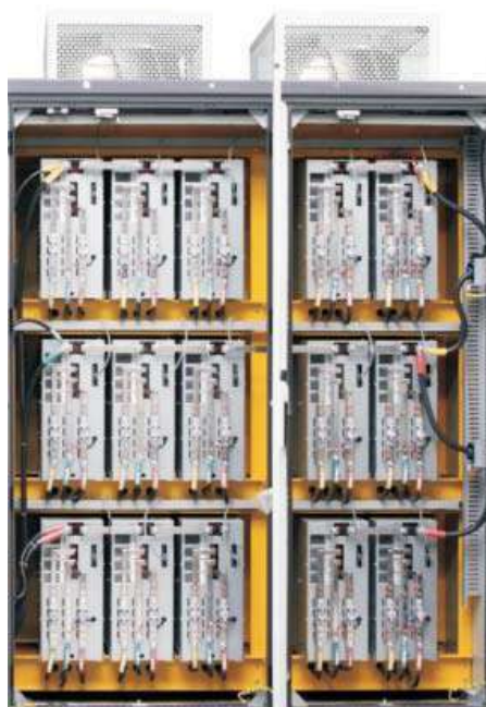
Fig 3.7 Layout in the power unit cabinet
