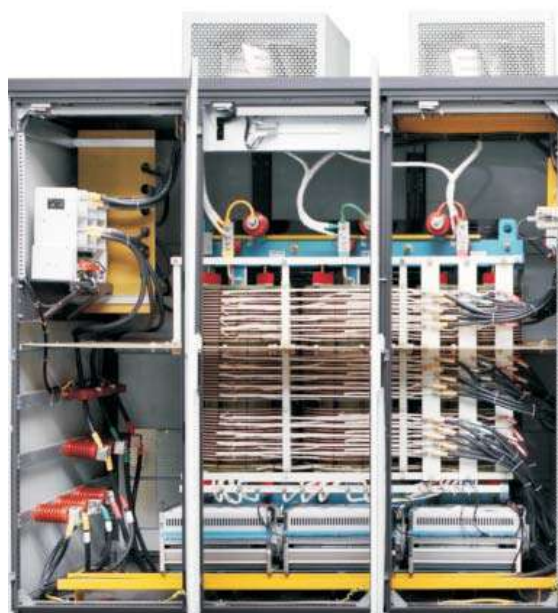
Fig 3.6 Layout in the transformer cabinet
